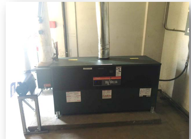
Cuyamaca College Building C New Boiler
